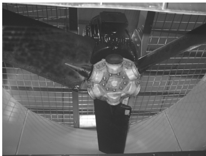
Figure 13: Axial Fan on Direct Drive Unit
